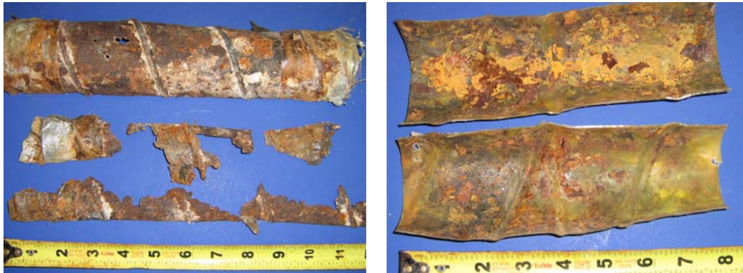
Figure 5.30: Beam 2.1 Duct Splices-South Duct Industry Standard Splice (Left) and North Duct Heat Shrink Splice (Right)
