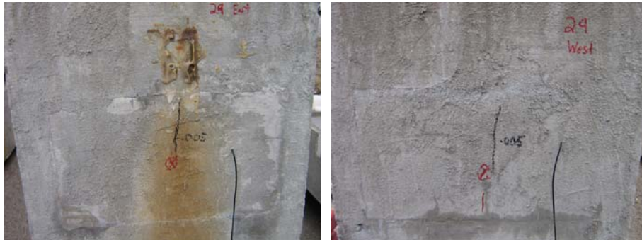
Figure 5.88: Beam 2.9 Anchorage Zones-East End (Left) with Dripper, and West End (Right) Without Dripper
