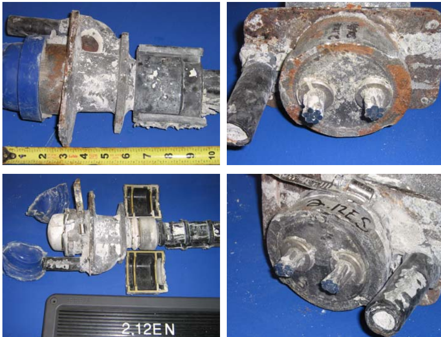
Figure 5.111: Beam 2.12 East End Anchorages (Dripped End)-South Duct Anchorage (Top, Left and Right), and North Duct Anchorage (Bottom, Left and Right)
