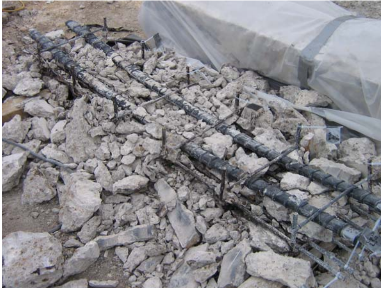
Figure 5.10: Post-Tensioning Ducts Before Removal From Center Block (Phase II Beam 2.12 Pictured)
