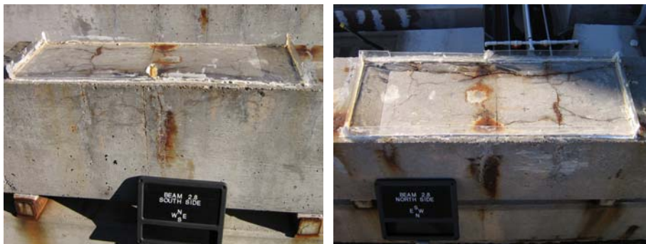
Figure 5.77: Beam 2.8-Side View (Left) and Top View (Right)-Note: These Views are from Opposite Sides of the Beam
