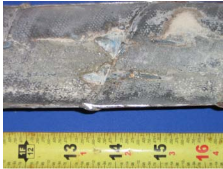
Figure 5.65: Beam 2.7-Evidence of Abrasion of Epoxy Coating from Strand on Bottom of South Duct
