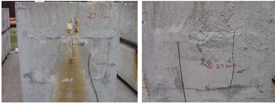
Figure 5.71: Beam 2.7 Anchorage Zones-East End (Left) with Dripper, and West End (Right) Without Dripper
