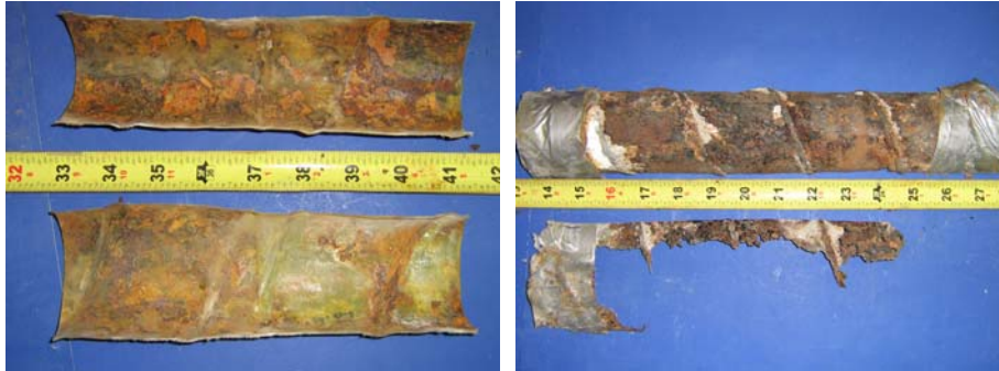
Figure 5.79: Beam 2.8 Duct Splices-South Duct Heat Shrink Splice (Left) and North Duct Industry Standard Splice (Right)
