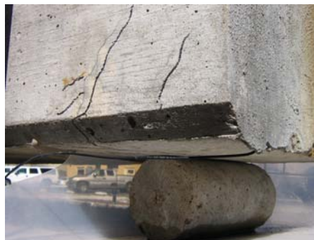
Figure 5.89: Beam 2.9: Bottom Corner of East End Anchorage Zone
