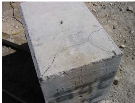
Figure 5.107: Beam 2.12-Cracking in East End Anchorage Zone
