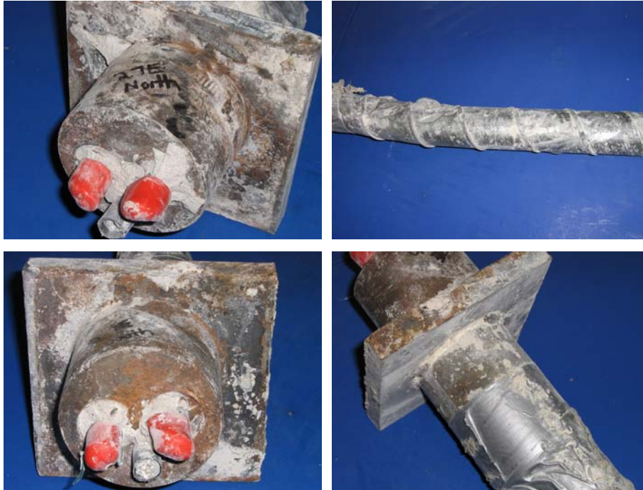
Figure 5.74: Beam 2.7 East End Anchorages (Dripped End): North Duct Anchorage (Top, Left and Right), and South Duct Anchorage (Bottom, Left and Right)
