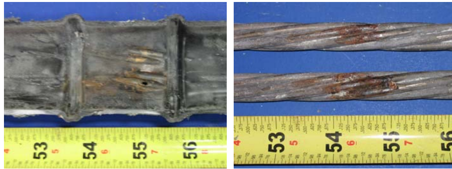
Figure 5.103: Beam 2.12-Abrasion Damage to Interior of North Duct (Left) and Strand From Same Location (Right)
