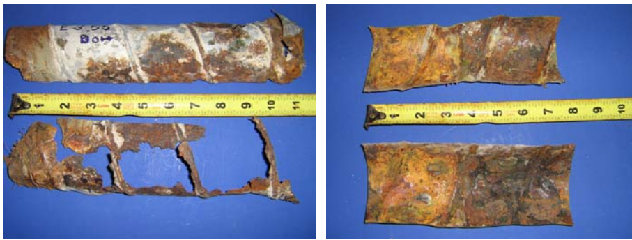
Figure 5.54: Beam 3.5 Duct Splices-South Duct Industry Standard Splice (Left) and North Duct Heat Shrink Splice (Right)
