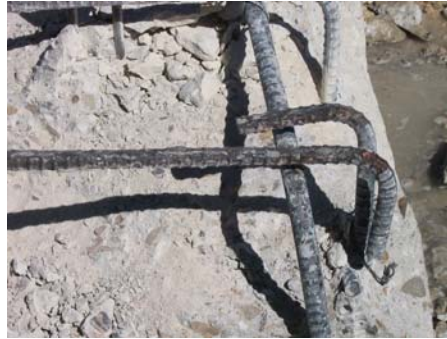
Figure 5.110: Beam 2.12-Corroded Stirrup in East End Anchorage Zone (Dripped End)
