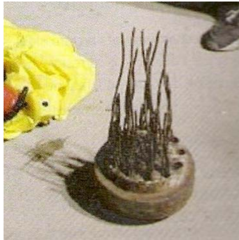
Figure 1.2: Corroded Anchorage (Bearing Plate with Strand Tails) 7
