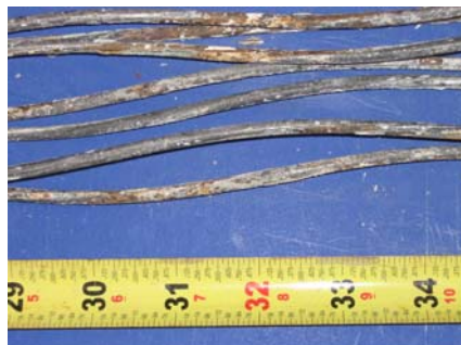
North Duct Galvanized Strand
