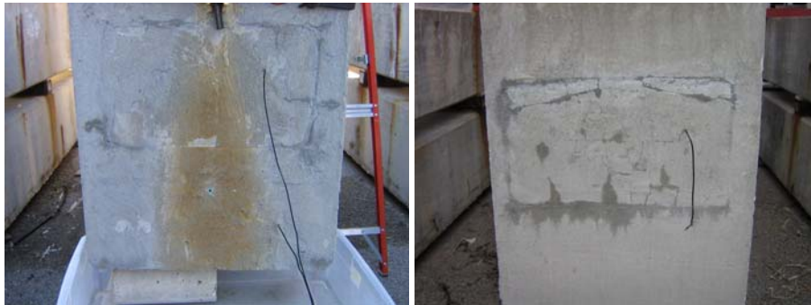
Figure 5.106: Beam 2.12 Anchorage Zones: East End Anchorage With Dripper (Left) and West End Anchorage Without Dripper (Right)
