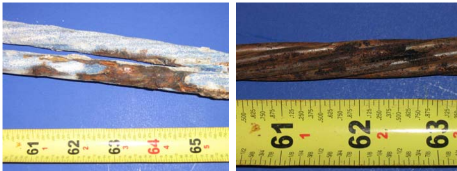
Figure 5.66: Beam 2.7-South Duct Strand With Coating (Left) and After Removal of Coating (Right)
