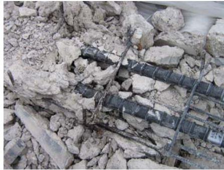
Figure 5.102: Beam 2.12 During Autopsy
